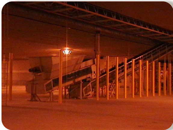
Belt Conveyors System
