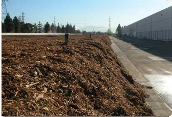
Biofilter at Inland Empire Regional Composting Facility After Media Placement
