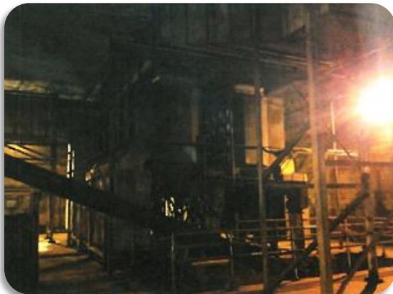
Dust Collection Fans
