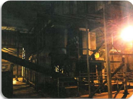
Dust Collection Fans
