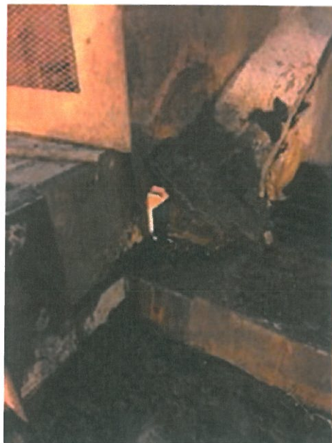
Biosolids hopper before repair
