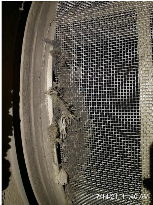
Screen cloth failure due to manufacturer design error
