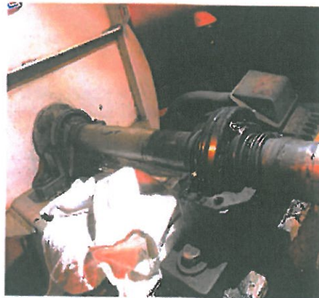
Bearing before repair
