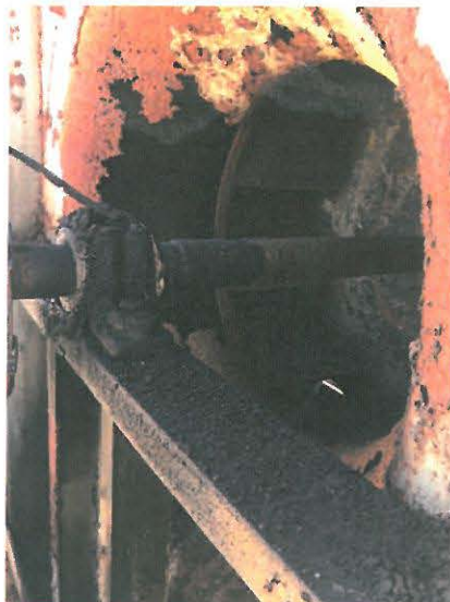
Corroded supply fan
