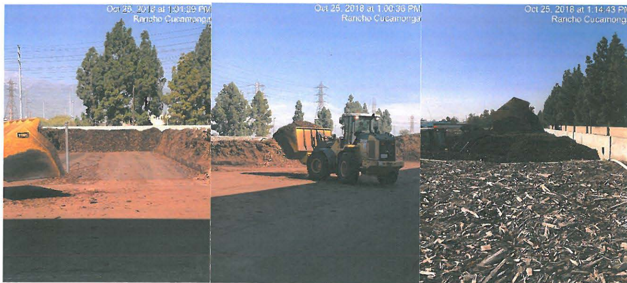
Biofilter media maintenance
