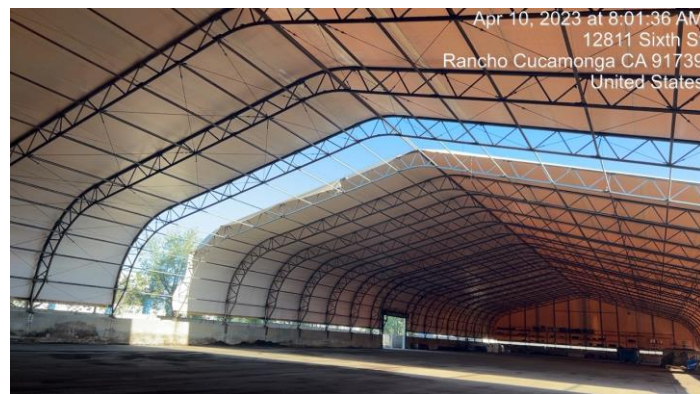
Storage Facility Tent Failing
