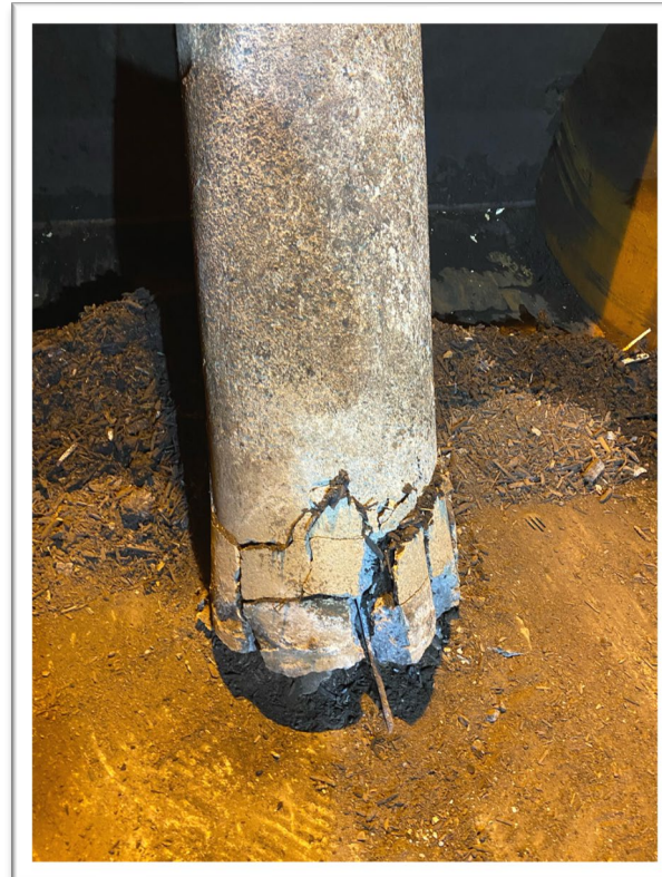
Column Before Repair
