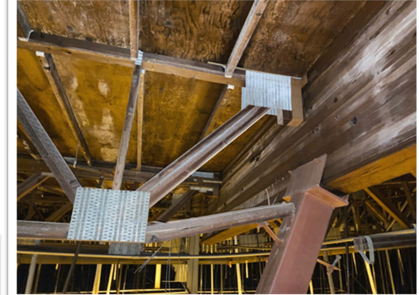
Damaged Glulam Beams
