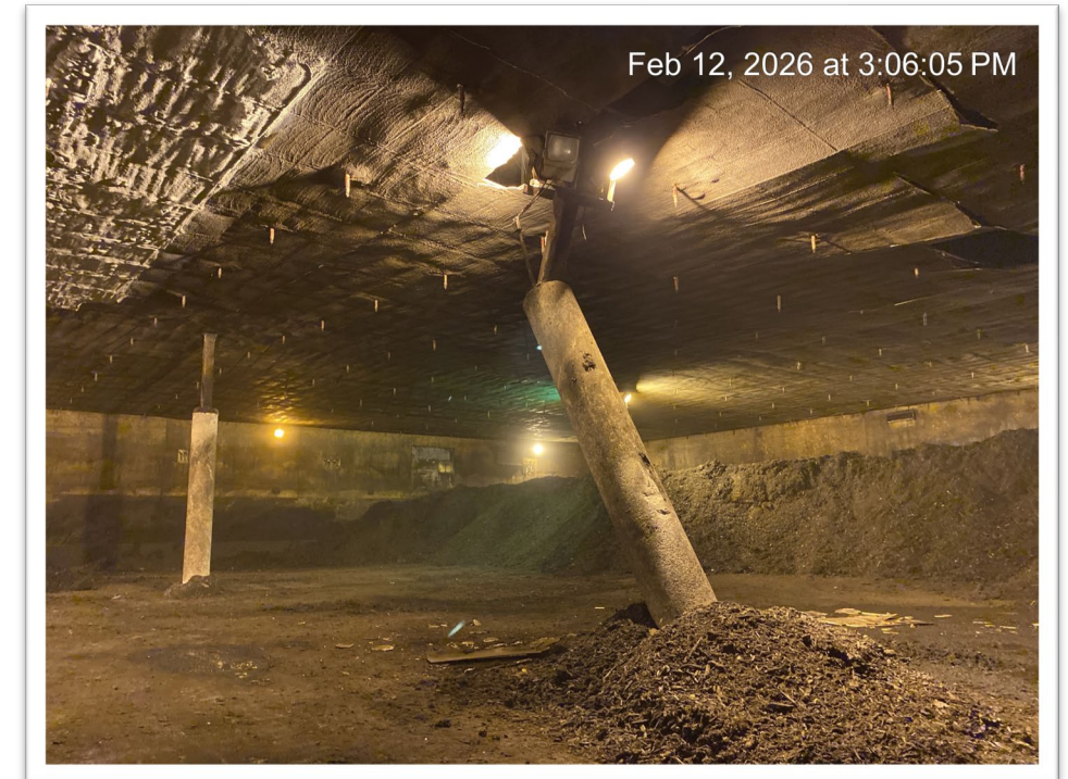
Structural Column Damage
